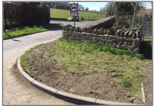
TIDY UP PATCH UP: Toll Down corner
